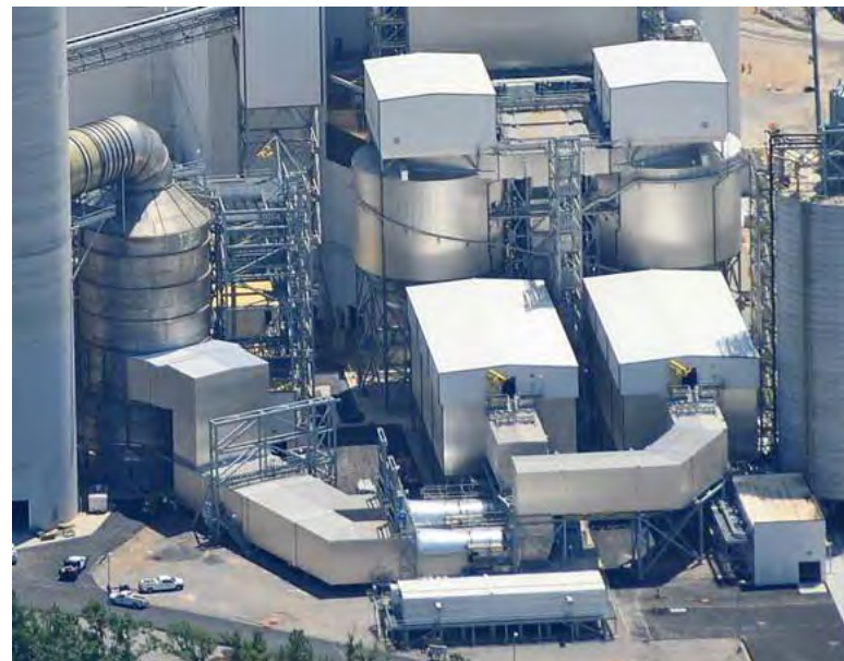
Duke Energy Cliffside Unit 6 Cliffside, NC
